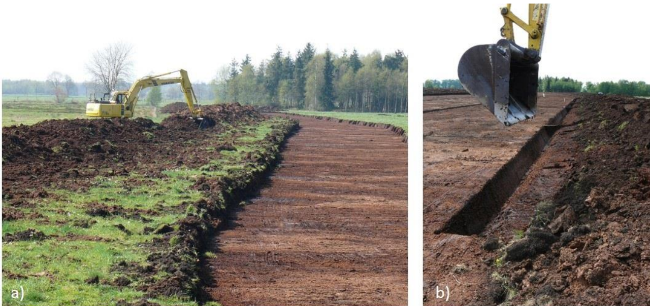
Figure 3. Setting up a Sphagnum farming site on former bog grassland in Germany (Rastede), using an excavator for a) removal of the degraded topsoil and b) construction of causeways and irrigation ditches. Photos: Sabine Wichmann.
